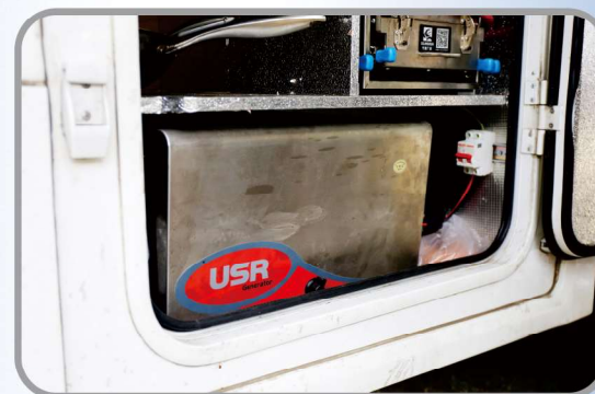
Type C RV installation
